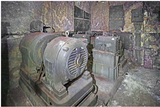
Two 3.5 kVA motor alternators (rotary converters) are seen in the radar machine room. This is now the only ROTOR site where these survive
